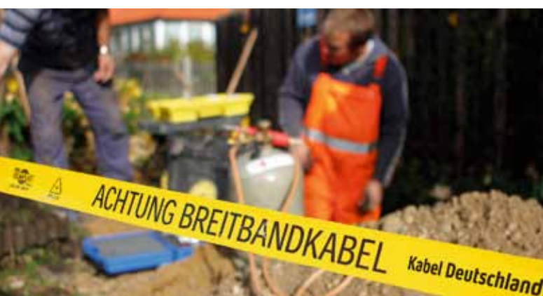
Under construction: Kabel Deutschland is upgrading many of the monofunctional TV lines throughout Germany so its customers can tap into state-of-the-art TV, broadband internet and telephony from a single outlet.
